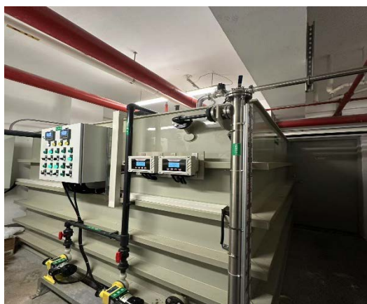
Photo: High-concentration Wastewater Collection Tank
